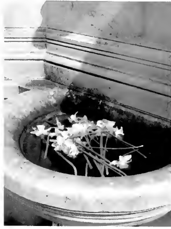
Figure 35: Pedestal basins do not drain and collect water and debris
